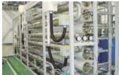
RO system (Toyooka Factory)
