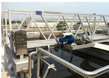
Reusing wastewater for cooling water (Hangzhou Yamaha)
