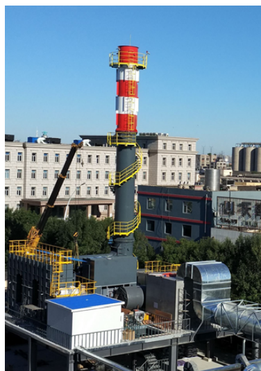
Yamaha's VOC disposal facility in Tianjin
