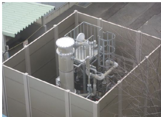
Groundwater purification equipment at the headquarters office
