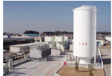
Cogeneration equipment at Kakegawa Factory
