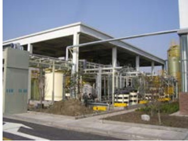
Wastewater treatment facility
