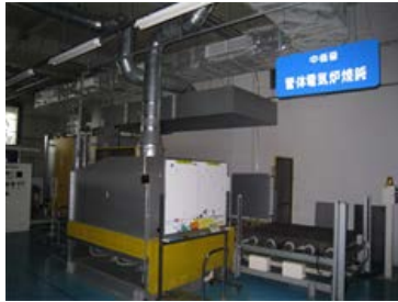
An upgraded electric annealing furnace
