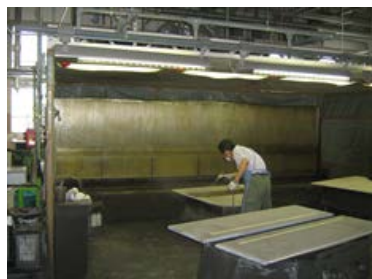
Wet painting booth(Kakegawa Factory)
