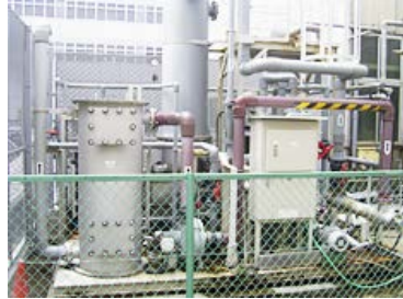
Groundwater purification equipment at the Headquarters Factory
