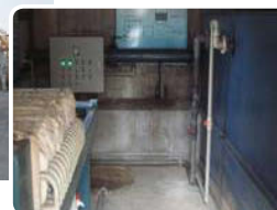
▲ Wastewater treatment equipment (Tianjin Yamaha Electronic Musical Instruments, Inc.)
