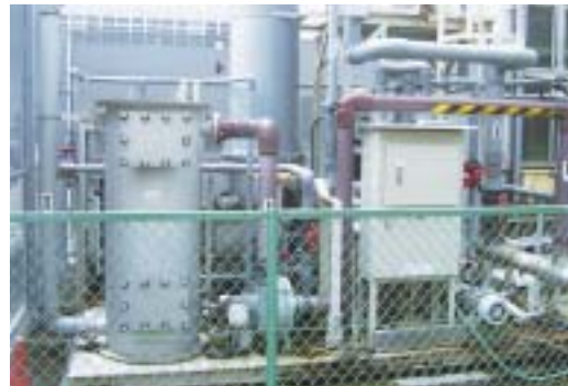
Groundwater purification equipment at the factory in the Yamaha Corporation's headquarters complex
