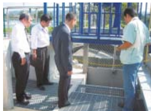
Automatic Shutdown Device on the Factory Wastewater Outlet
