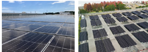
Solar panels installed at the Kakegawa Factory
