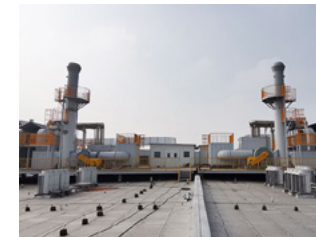
VOC treatment facility (Hangzhou Yamaha Musical Instruments)
