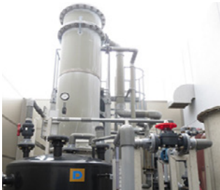
Groundwater purification equipment at our headquarters
