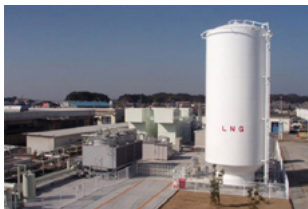
Cogeneration system at the Kakegawa Factory
