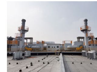
VOC treatment facility (Hangzhou Yamaha Musical Instruments)
