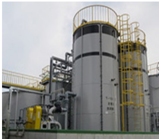
Wastewater processing equipment at the Toyooka Factory
