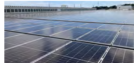
Solar panels installed at the Kakegawa Factory
