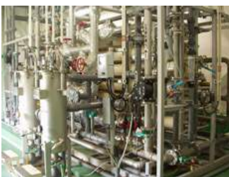
Reverse osmosis (RO) membrane device (Toyooka Factory)
