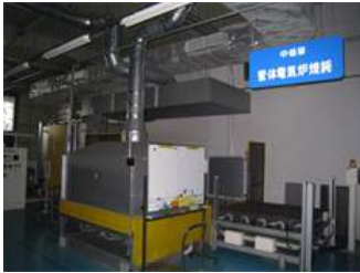
An upgraded electric annealing furnace
