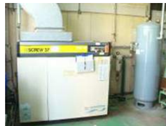
Compressor in which the pressure has been set at an appropriate level
