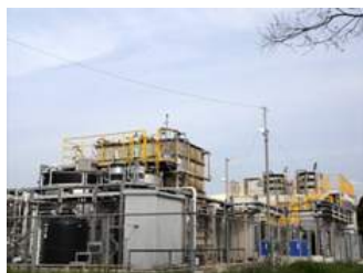
Wastewater treatment facility at the Takegawa Factory
