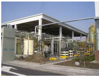
Wastewater treatment facility (Xiaoshan Yamaha)
