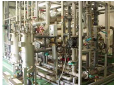
Reverse osmosis (RO) membrane device(Toyooka Factory)
