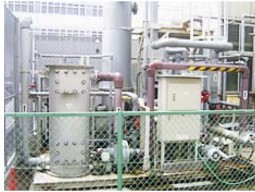
Groundwater purification equipment at the Headquarters Factory
