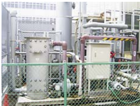
Groundwater purification equipment at the factory at Yamaha headquarters
