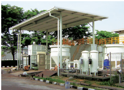
The upgraded water treatment facilities
