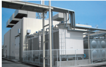
The cogeneration system installed through the ESCO.
