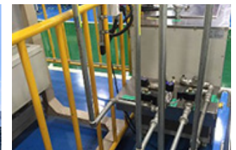
Cooling unit using circulated water
