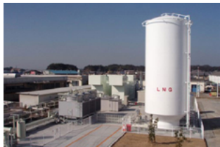
Cogeneration system at Kakegawa Factory
