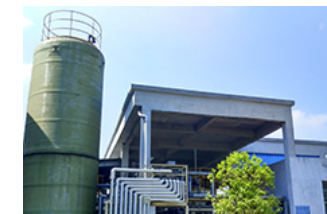
Wastewater treatment facility
