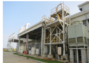
Wastewater treatment facility
