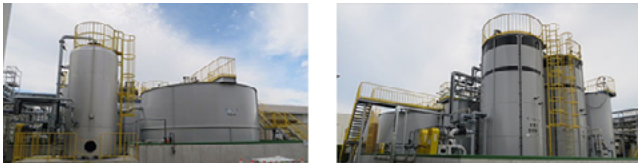
Wastewater processing equipment at the main factory of Yamaha Music Manufacturing Japan
