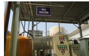
Reverse osmosis membrane equipment
