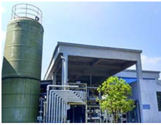
Wastewater treatment facility (Xiaoshan Yamaha Musical Instrument Co., Ltd.)
