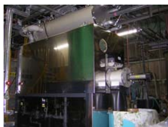
Vacuum concentration equipment (Toyooka Factory)
