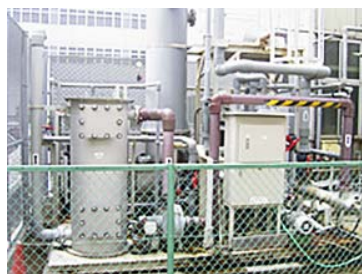
Groundwater purification equipment at the headquarters office
