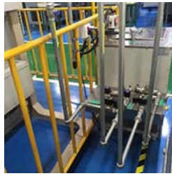
Cooling unit using circulated water (Xiaoshan Yamaha Musical Instrument Co., Ltd.)
