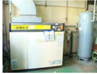
Compressor in which the pressure has been set at an appropriate level
