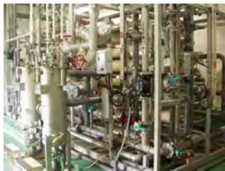
Reverse osmosis (RO) membrane device (Toyooka Factory)
