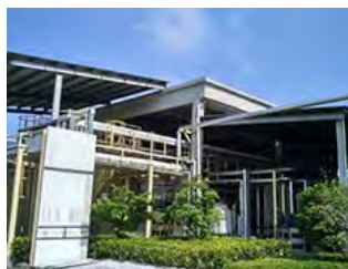
Wastewater treatment facility2 (Xiaoshan Yamaha)
