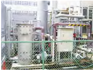
Groundwater purification equipment at the headquarters business site
