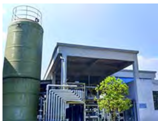
Wastewater treatment facility1 (Xiaoshan Yamaha)
