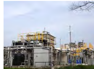
Wastewater processing facility (Kakegawa Factory)
