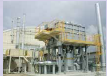
Regenerative exhaust-gas heat treatment system
