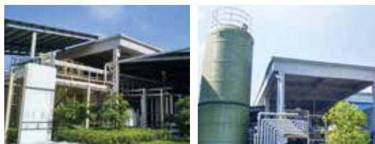
Cooling unit using circulated water
