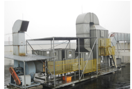
VOC treatment facility at Xiaoshan Yamaha Musical Instruments Co., Ltd.
