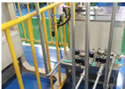
Cooling unit using circulated water
