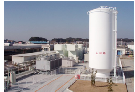
Cogeneration system at Kakegawa Factory
