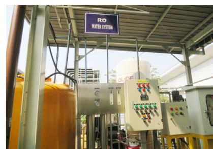
Reverse osmosis membrane equipment
