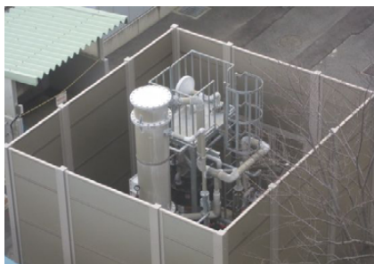
Groundwater purification equipment at the headquarters office
