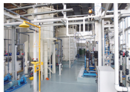
Reuse of 100% of manufacturing process wastewater
