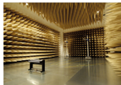
Anechoic chamber used for electromagnetic wave measurement
