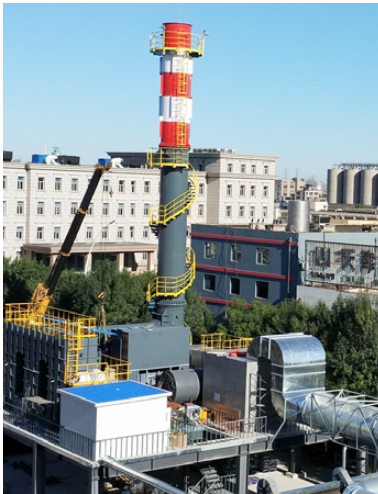
VOC treatment facility at Tianjin Yamaha Electronic Musical Instruments, Inc.
