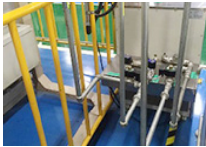
Cooling unit using circulated water
