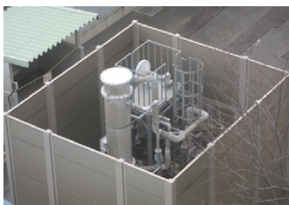
Groundwater purification equipment at the headquarters office
