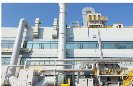
Yamaha's VOC disposal facility in Hangzhou
