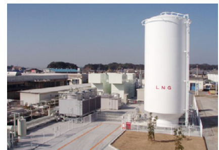
Cogeneration equipment at Kakegawa Factory
