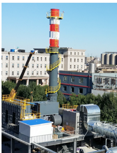
Yamaha's VOC disposal facility in Tianjin
