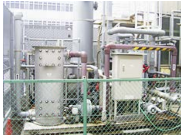
Groundwater purification equipment at the Headquarters Factory
