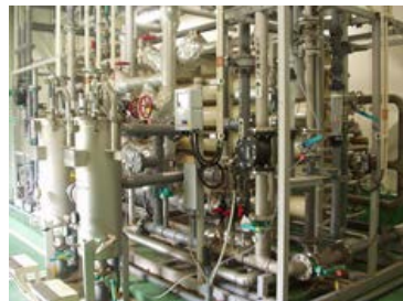
Reverse osmosis (RO) membrane device (Toyooka Factory)
