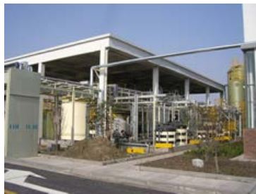
Wastewater treatment facility
