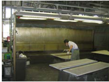
Wet painting booth(Kakegawa Factory)
