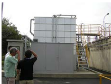
Additional wastewater treatment equipment
